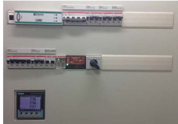
Above: Part of LDB with LPM and Power Meter
